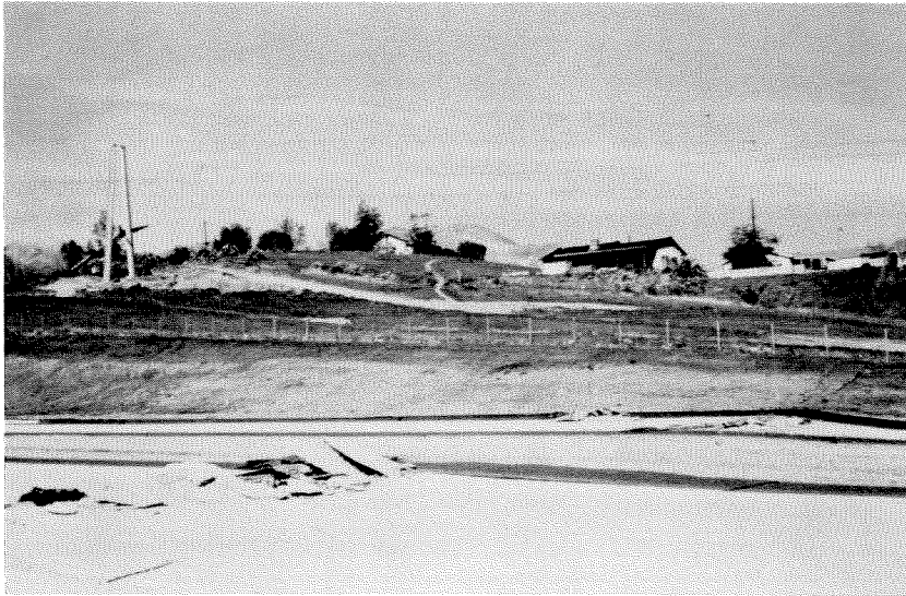
Figure 6.79 Pavement damage from surface faulting. Foothill freeway northwest of Maclay Street.
