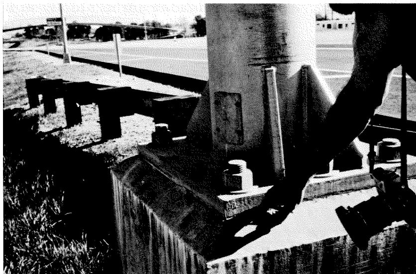
Figure 7.42 Base of the Polk Street exit sign shown above. Spalled concrete indicates small movements at the base of the undamaged structure.
