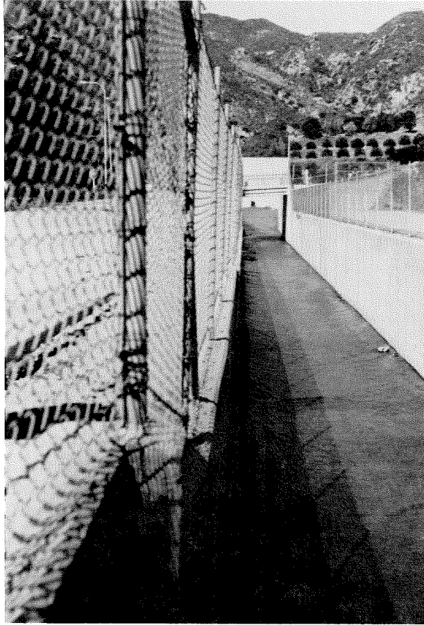
Figure 4.22 Motion of retaining wall of flood control channel towards channel. Joint in foreground has displaced about 4 inches; joint in middle distance about 2 inches. Near Olive View Hospital.
