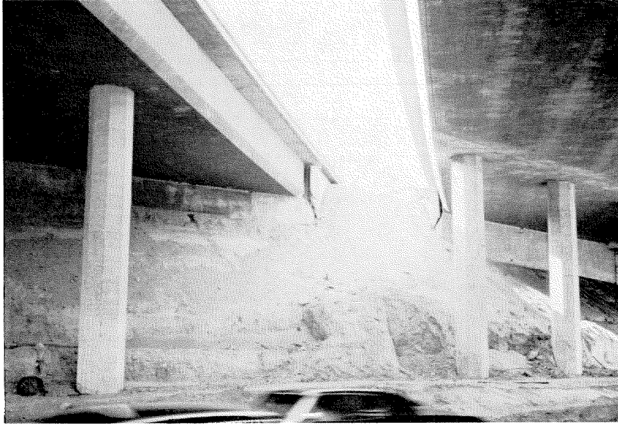
Figure 6.90 Damage to the northern abutment of the West Sylmar Overhead, Golden State freeway.
