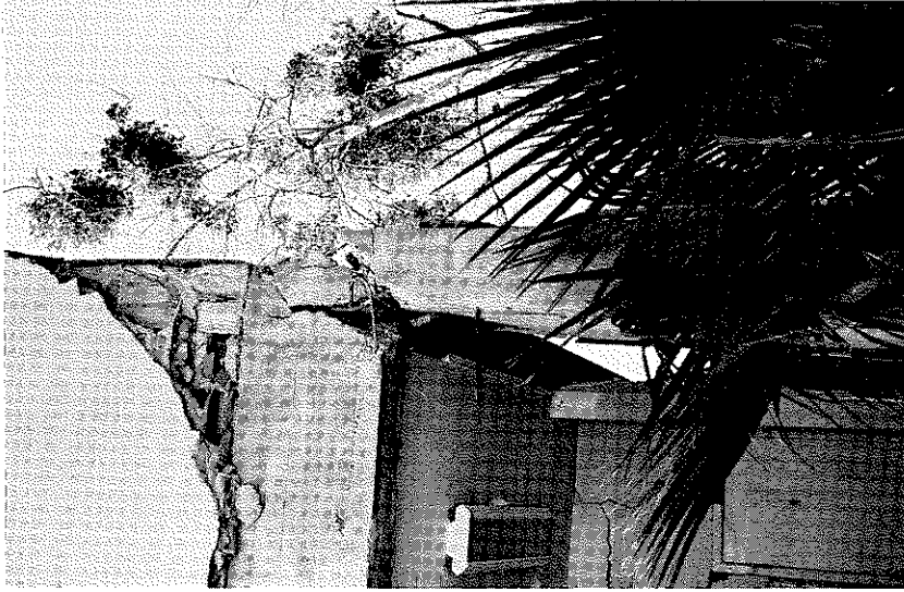
Figure 3.49 Eastern corner of the Men's Ambulant Building, Veterans Hospital, showing column damage.
