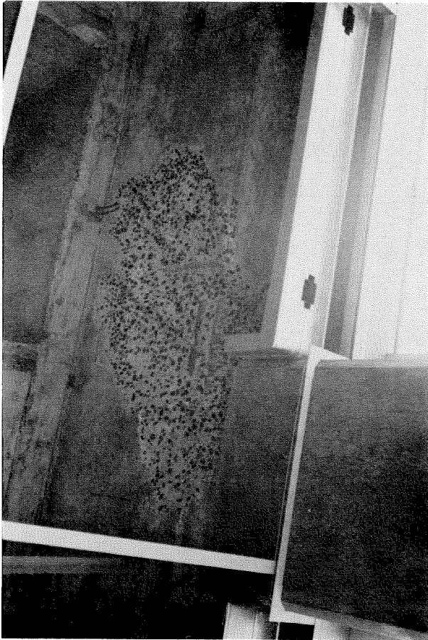
Figure 3. 156 The concrete cracked and spalled in the region of the beam-column connection with no visible damage to the reinforcing steel, fourth floor level, Bank of California.
