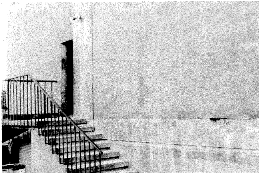
Figure 3.135 Cracking and spalling on the construction joint above the first floor slab. Lightweight concrete was used for the slab and beam construction. Nethercutt Museum.
