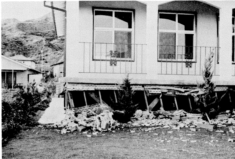
Figure 3.183 A house on Aldergrove Street that shows horizontal movement on its wood supports.
