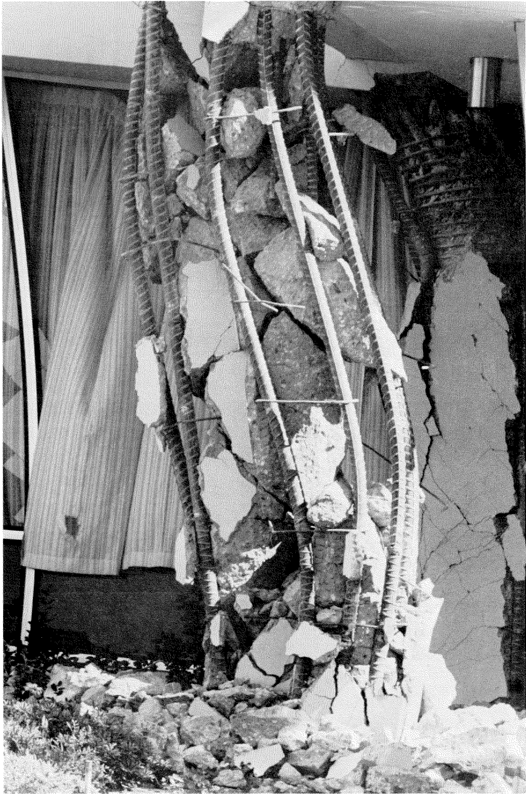
Figure 3.24 Shattered L-shaped corner column, Olive View Hospital. The ties are No. 3's at 18 in on centers.
