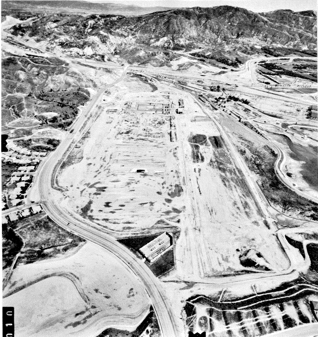
Figure 1.21 Aerial view looking N 27° W across Metropolitan Water District Balboa Water Treatment Plant site. The settling basins are in the background and the rectangular outline of the underground reservoir can be seen just this side of the contractor's work area. The small dark rectangle is a portion of the south edge of the reservoir not yet covered. Balboa Blvd. is on the left-hand side of the site, upper Van Norman Reservoir is on the right-hand side, and the Pacific Intertie Converter Station and the San Fernando Juvenile Facility are just beyond. The old San Fernando Electric Power Plant is in the small white building between the Intertie and the settling basins. In the center foreground is the Balboa Blvd. electrical switching station of the Los Angeles Department of Water and Power where cantilevered concrete walls were damaged by the earthquake.
