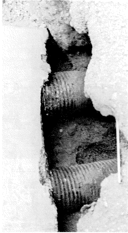
Figure 6.57 Piling damage at the western abutment of the southern bridge, Roxford undercrossing of the Foothill freeway.
