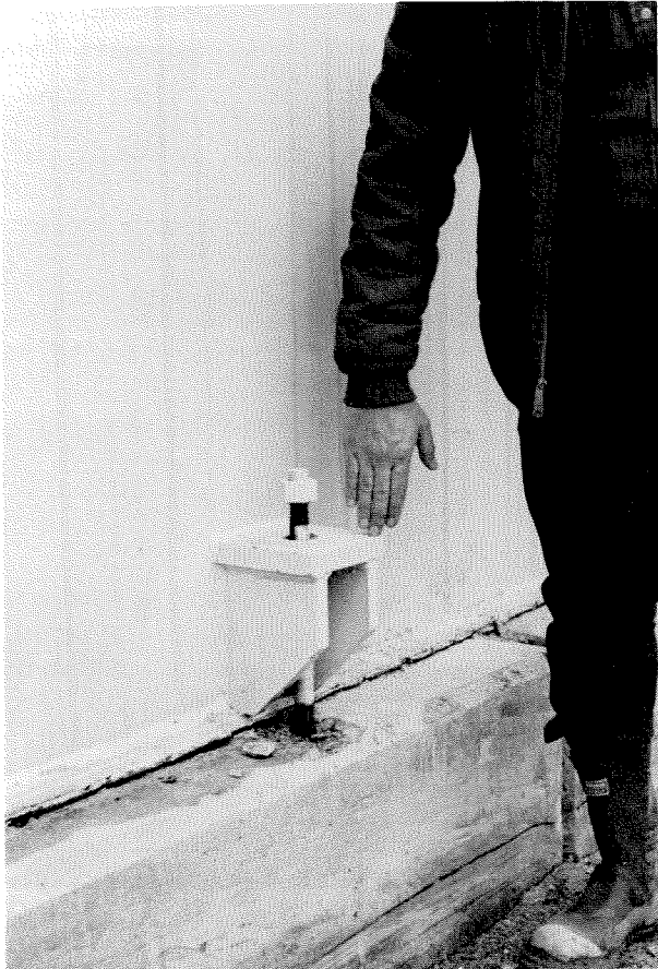
Figure 7.19 Anchor bolt pulled out; also shown in Figure 7.18.
