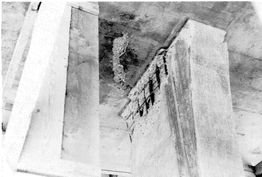
Figure 6.62 Column damage at the Bledsoe Street overpass, Foothill freeway.
