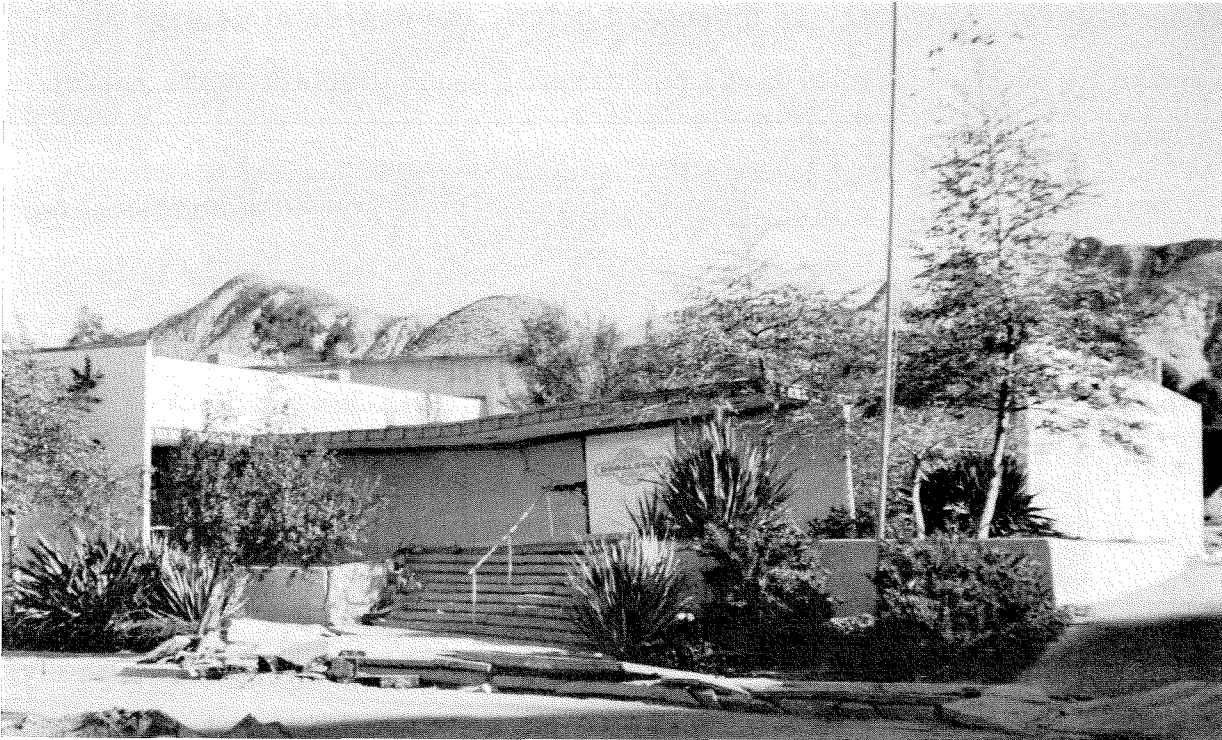
Figure 3.116 Structural damage resulting from permanent ground displacements. Donaldson Building.
