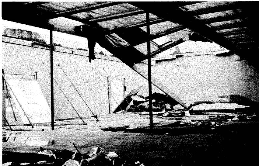
Figure 3.144 Collapse of a section of roof at the rear wall of the building shown in Figure 3.143. Laminated timber roof beams are supported at midspan by 6 in diameter steel columns.
