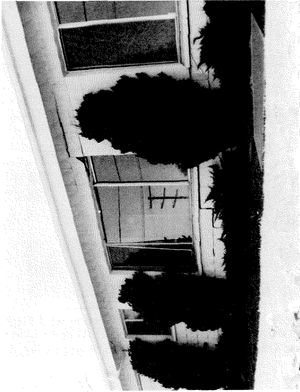
Figure 3.113 Structural damage to block walls, Foothill Nursing Home.
