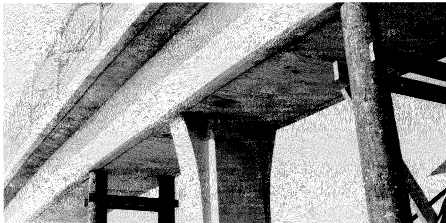
Figure 6.65 Damage to the tallest column of the Tyler Street footbridge, Foothill freeway.
