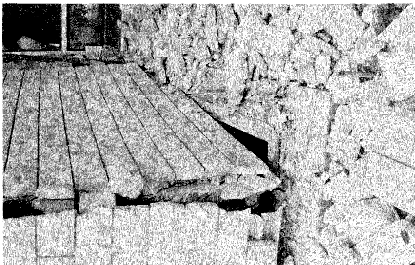
Figure 3.23 Exterior wall of elevator shaft moved about 16 inches to the north at the separation joint.
