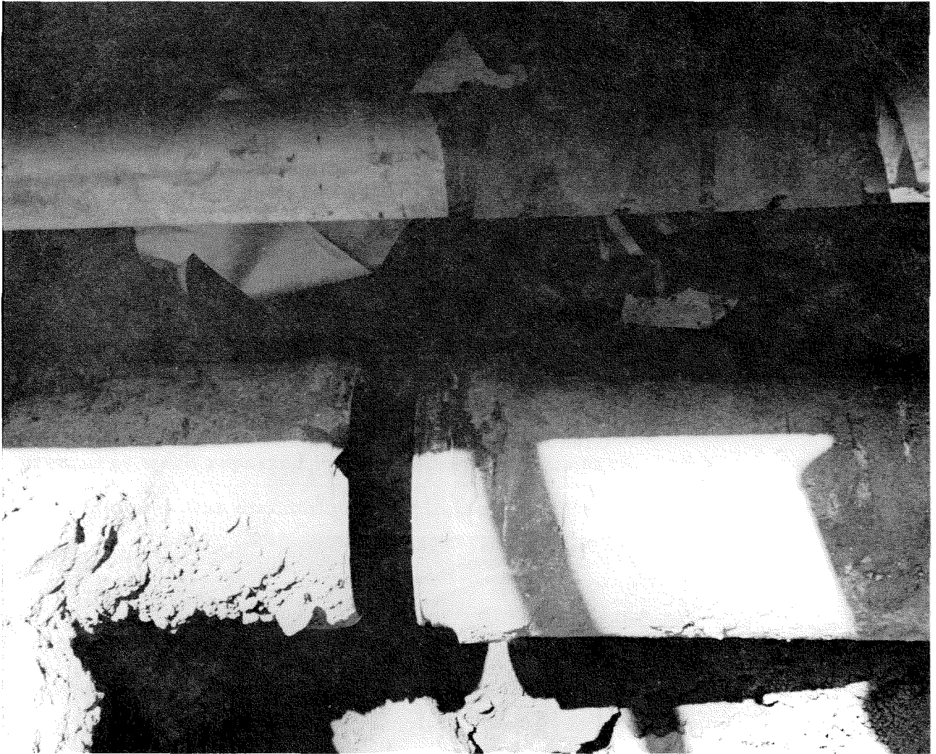
Figure 5.34. Underground pipes pulled apart on Glenoaks Street just southeast of Hubbard Street.
