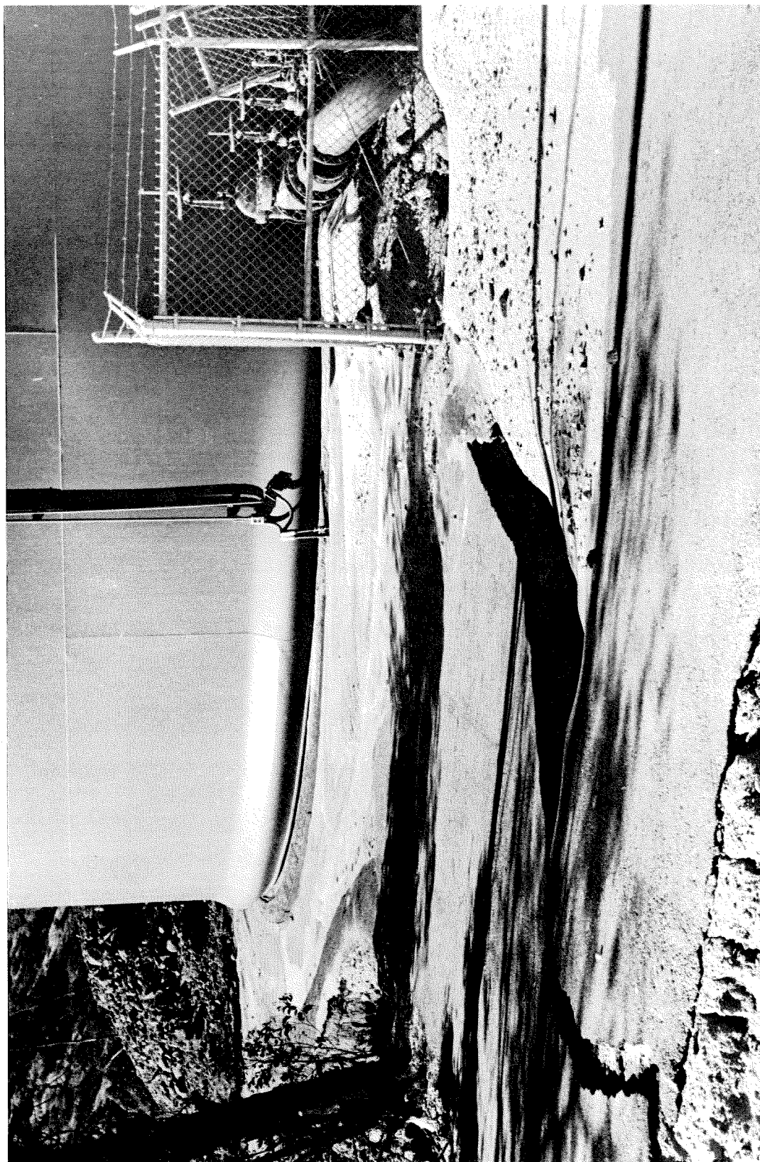
Figure 7.26 Water tank at Olive View Hospital. The vibrational damage caused failures of the tank base and adjoining piping, and the water was lost.
