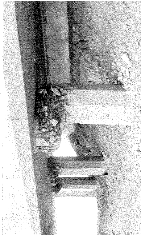
Figure 6.27 Column failures, northwest connector overcrossing, Golden State-Foothill freeway interchange.
