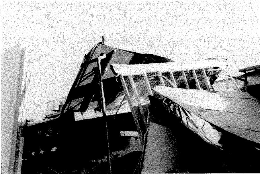
Figure 3.119 A section of collapsed roof showing the 1/2 in plywood, 11 in x 3-1/2 in purlins and steel connectors. Vector Electronics Building.
