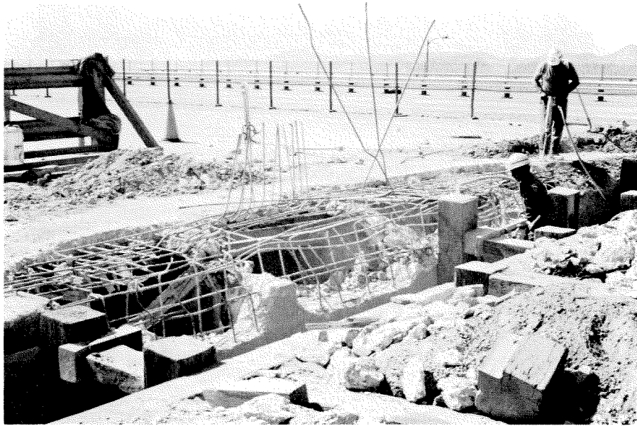
Figure 6.83 Concrete removal prior to repair of northern abutment of northbound lanes of Roxford Street undercrossing, Golden State freeway.
