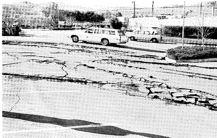
Figure 3.91 Evidences of ground movement in central parking area of the San Fernando Juvenile Facility.
