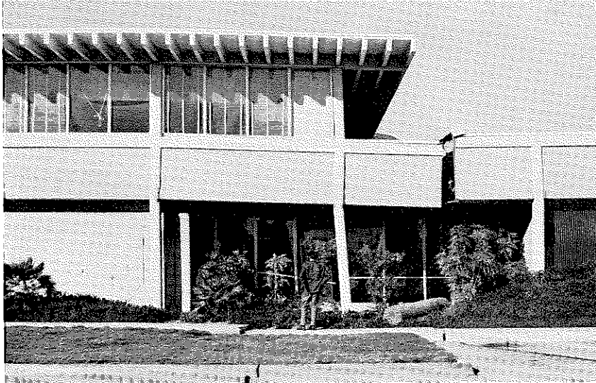
Figure 3.92 View showing ground displacements, reinforced concrete column failure, and opening of separation joint. San Fernando Juvenile Facility.
