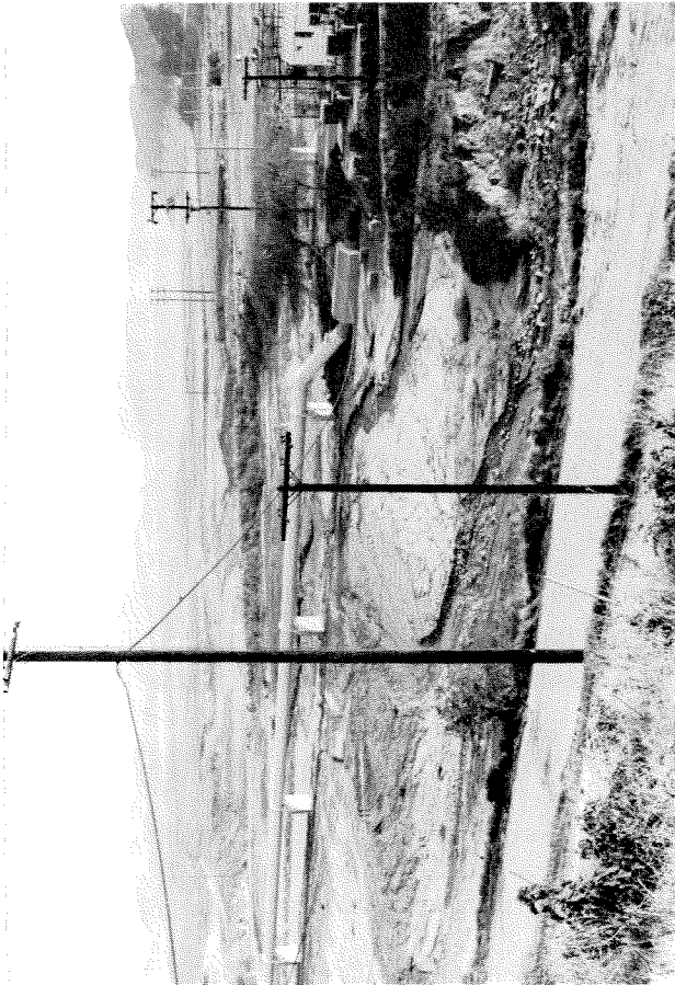
Figure 7.53 The supports of this steel water pipe, parallel to and just below upper Van Norman Dam had its supports deformed. The damage indicated a relative compression of the ground parallel to the pipe. The steel supports of the pipe underwent as much as several inches of deformation but the pipe was not damaged.
