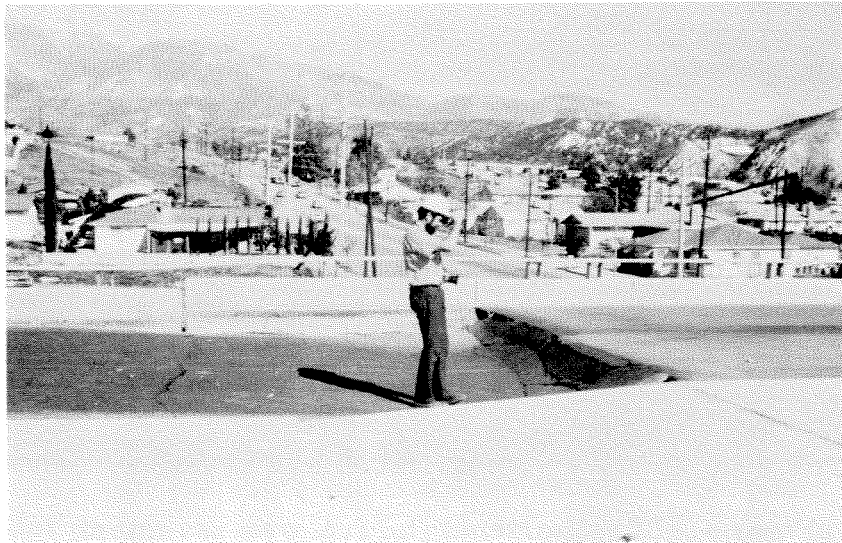
Figure 6.78 Settlement of abutment backfill, Maclay Street undercrossing, Foothill freeway.
