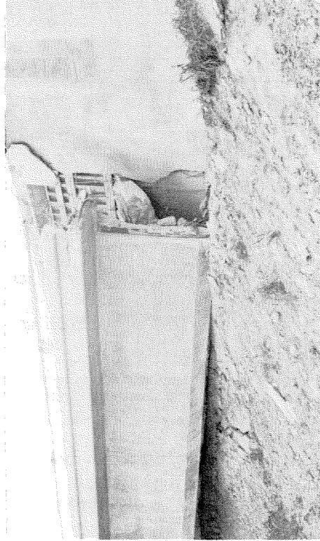
Figure 6.28 Northwest abutment of the northwest connector overcrossing, Golden State-Foothill freeway interchange.
