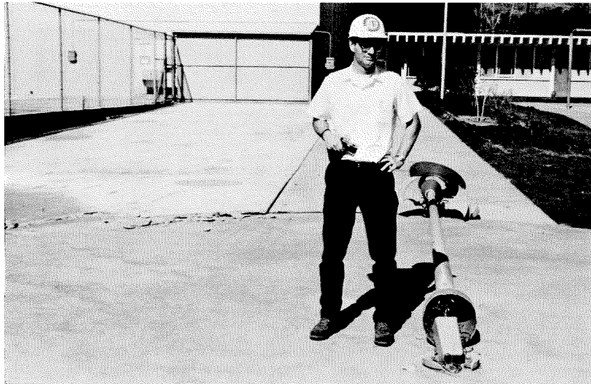
Figure 7.36 Collapsed light standard at the San Fernando Juvenile Facility.
