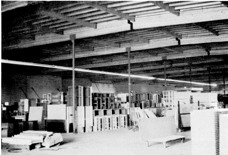
Figure 3.140 Interior view showing the roof structure and 6 in diameter steel supports. Sawyer Cabinet Inc. Building.
