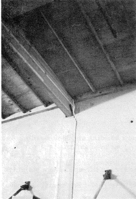
Figure 3.141 Detail of roof beam connection to tilt-up walls. The bracing at the middle of the walls was added after the earthquake. Sawyer Cabinet Inc. building.
