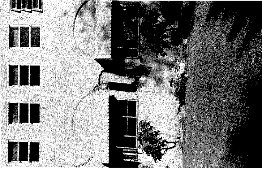
Figure 3.55 Shear failure of column, Infirmary Building (Bldg. 6), Veterans Hospital.
