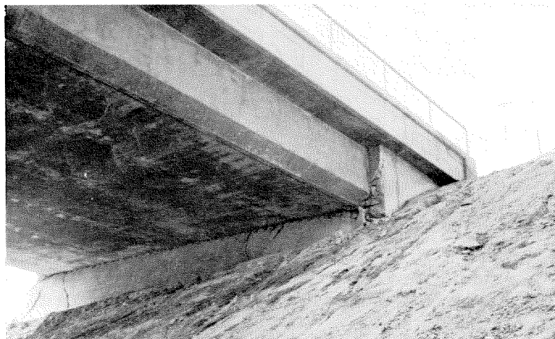
Figure 6.87 Northern face of the western abutment, Balboa Street overcrossing, Golden State freeway.
