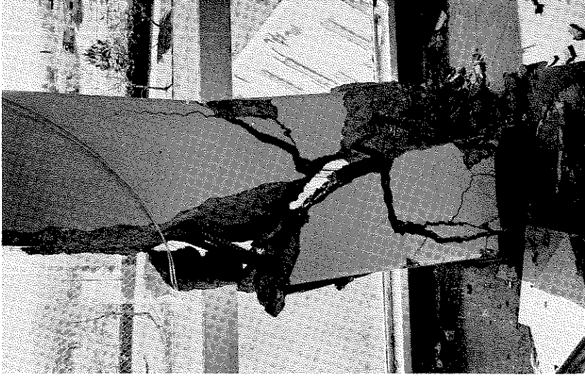
Figure 3.70 The third floor column between the end walls shown in Figure 3.69 was destroyed. Holy Cross Hospital.
