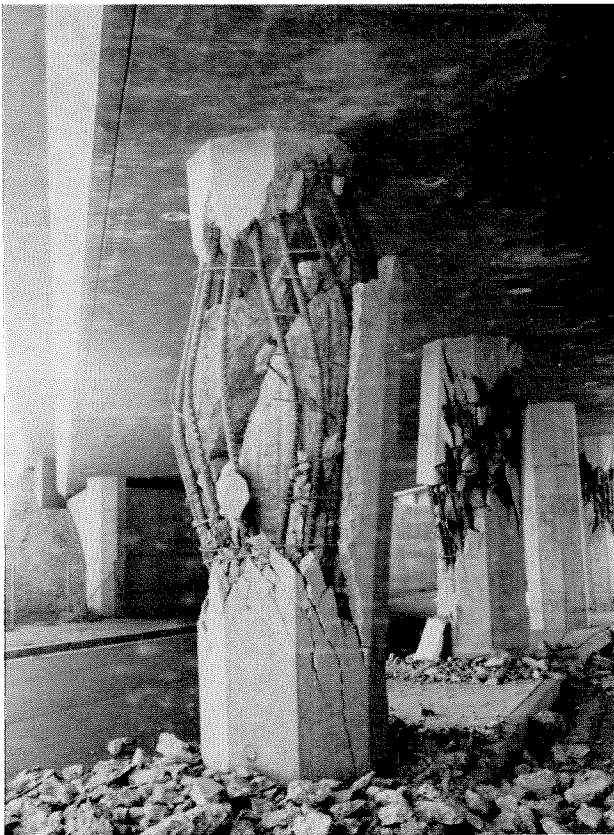
Figure 6.43 Failed columns of the southeastern bridge, Foothill Boulevard undercrossing, Foothill freeway.
