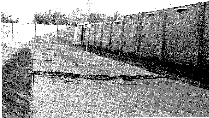
Figure 3.95 Ground displacement near northeast corner of San Fernando Juvenile Facility. The walls are concrete block construction.
