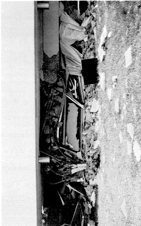
Figure 3.13 Destroyed column in Psychiatric Day Care Center, Olive View Hospital. The lightweight concrete shattered completely.
