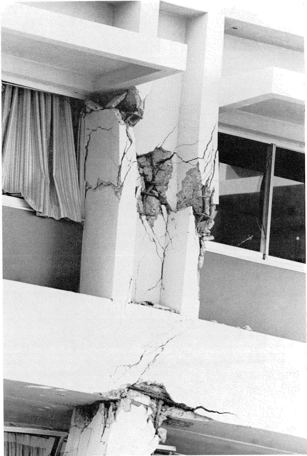
Figure 3.29 Shear failure in a second story column of the west wing, Olive View Hospital.
