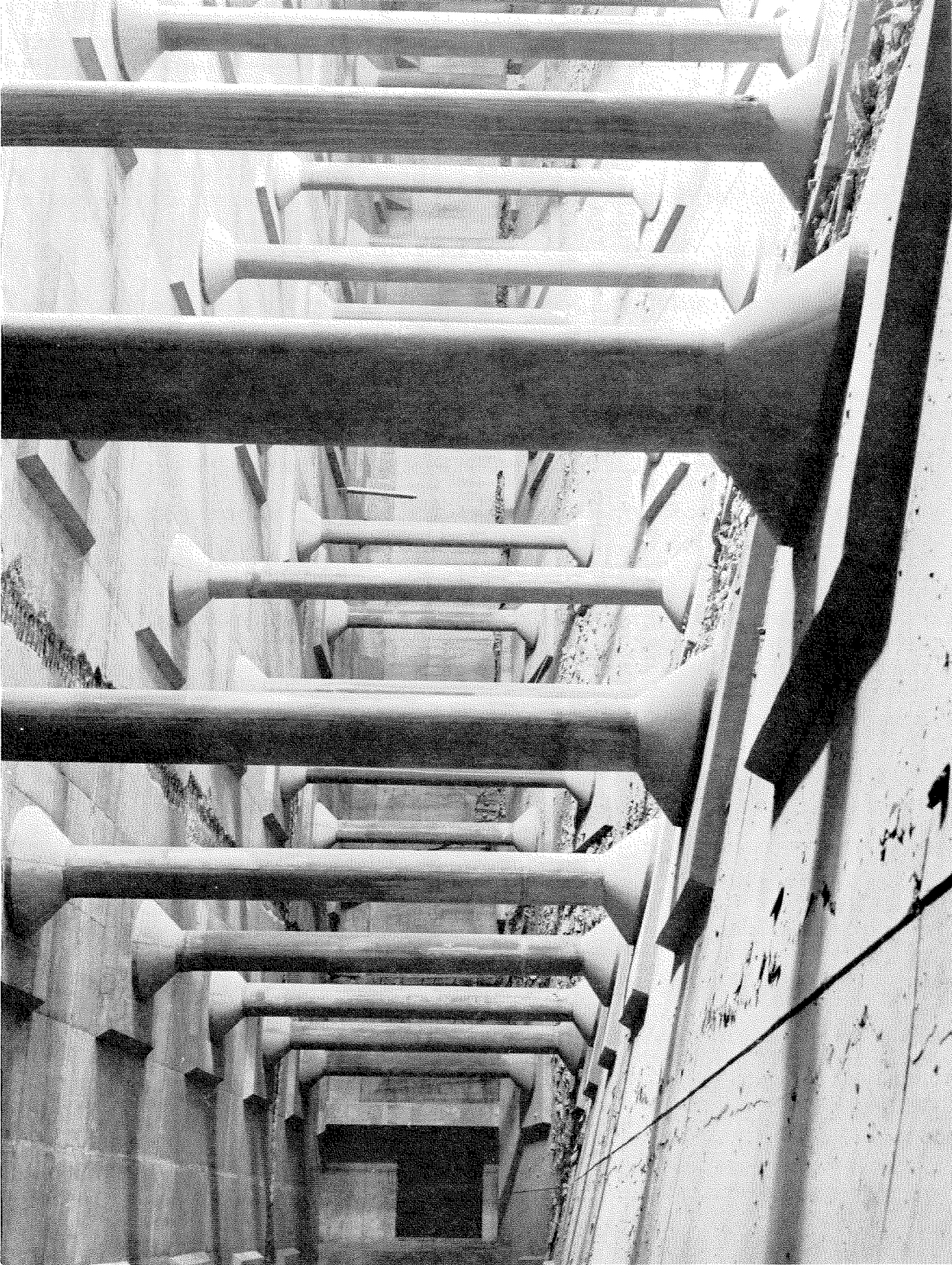
Figure 7. 9 Interior view of reservoir showing damage to roof slab, and what appears to be compression failure in floor slab along a construction joint. (MWD photograph).
