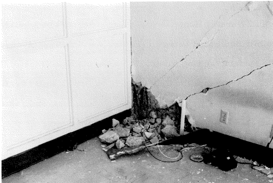
Figure 3.110 Interior view of the eastern shear wall of the three-story wing, Pacoima Lutheran Hospital.
