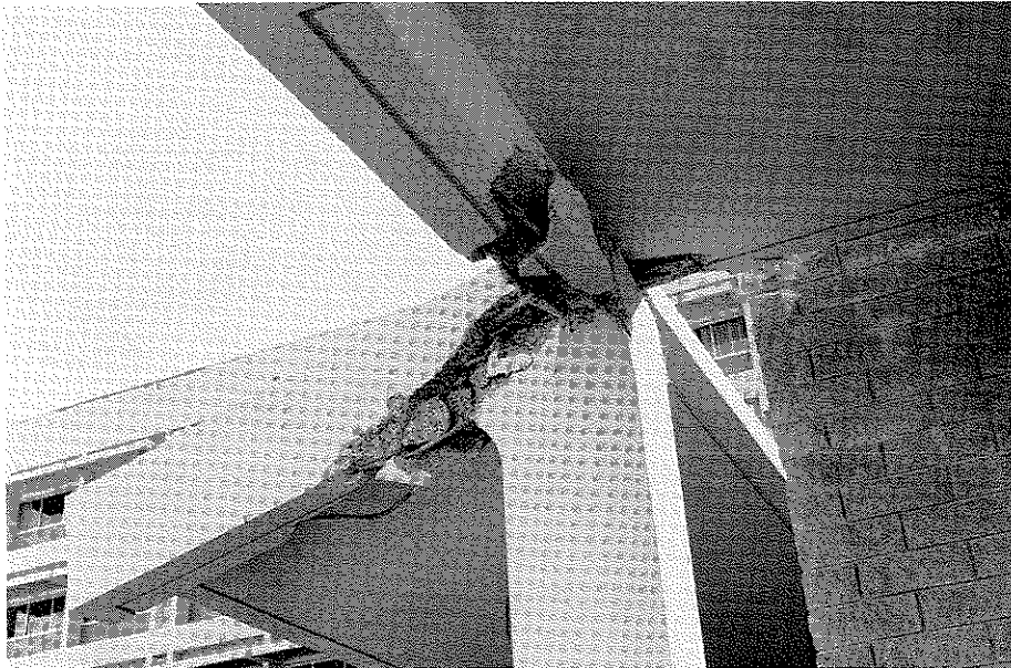
Figure 3.34 Beam and connection failure in the free-standing canopy of the exhaust pavilion, Olive View Hospital. The failure pattern suggests torsional failure of the beams from lateral motion of the structure. Note the scars on the brick facing of the separate, interior structure.
