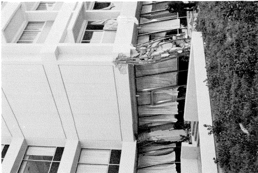
Figure 3.21 Shear wall at the north end of the southwest wing, Olive View Hospital.
