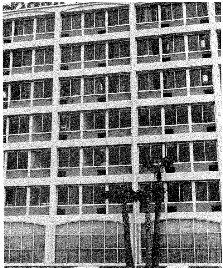
Figure 3.160 North elevation of building on March 21st. The second, third and fourth floors suffered severe non-structural damage estimated to be approximately $250,000. An aftershock seven weeks after the main earthquake damaged the repairs that had already been made.
