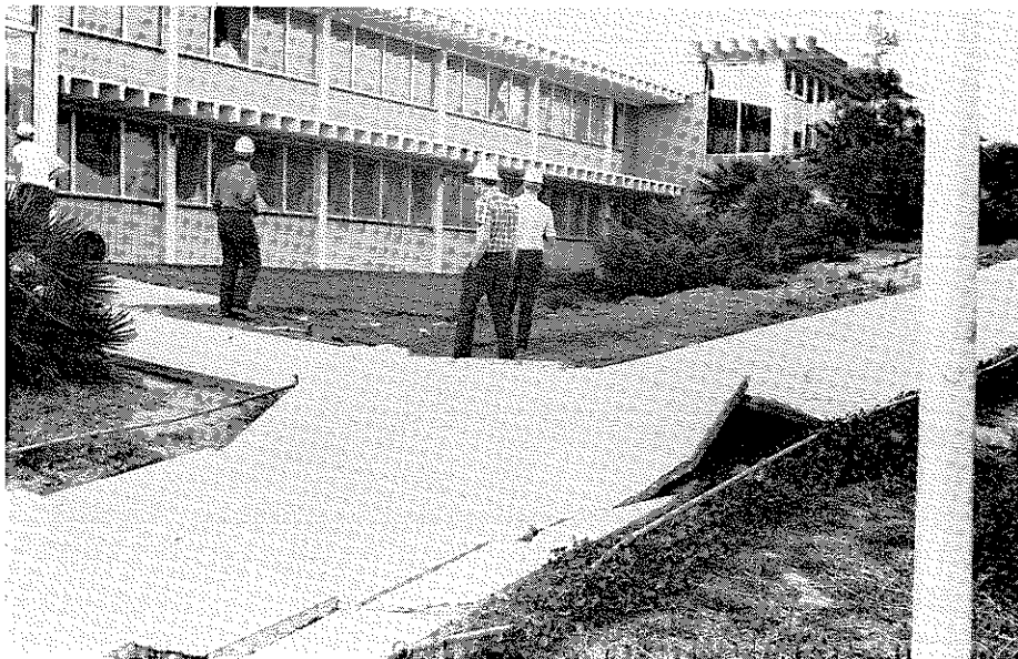
Figure 3. 97 Buckled sidewalk at San Fernando Juvenile Facility.
