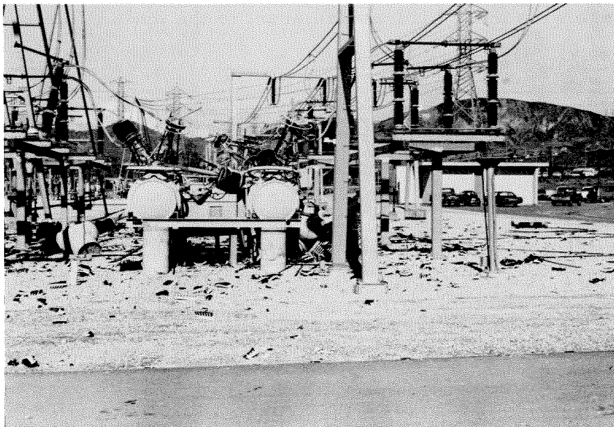
Figure 5.13 Air-blast circuit breakers, Sylmar Switching Station.
