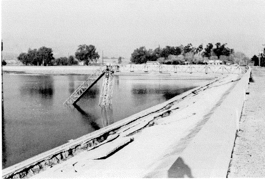
Figure 7.43 Collapsed elevated walkway at upper Van Norman Reservoir.
