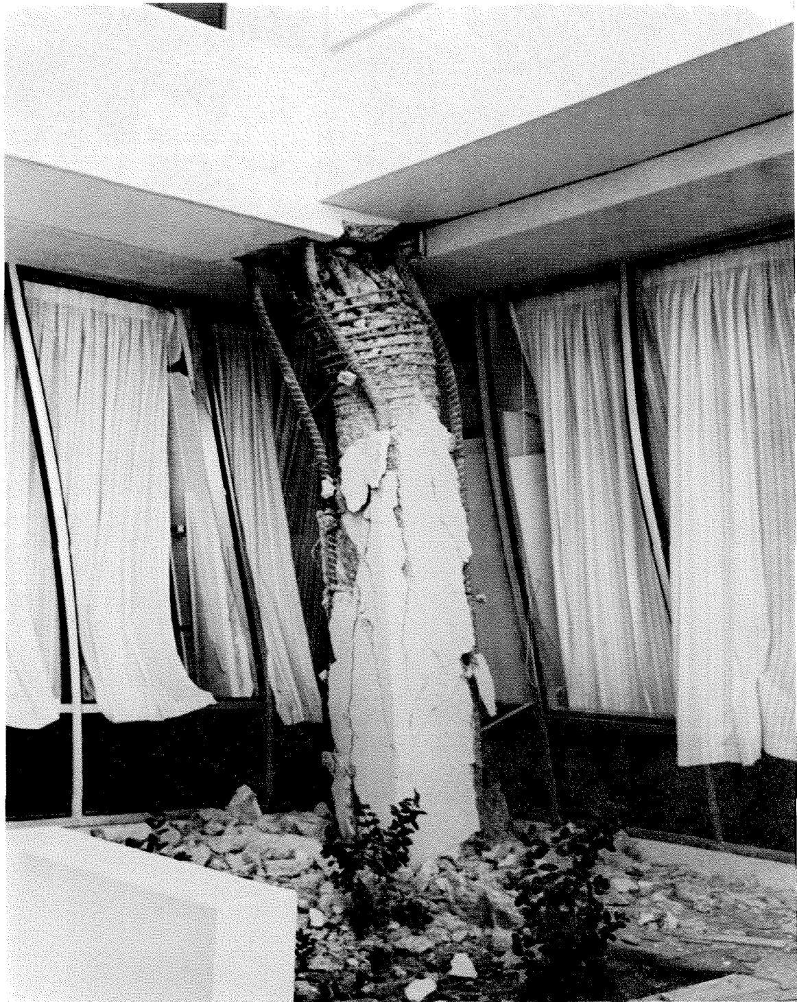
Figure 3.27 Damaged column at Olive View Hospital. This square concrete column had a circular, spirally wound core, and had four large bars outside the core at the corners. Those with tied outside bars performed somewhat better than those without ties shown in Figure 3.25.
