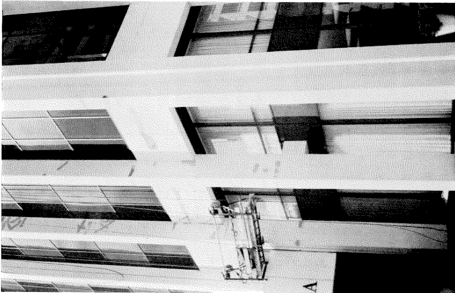
Figure 3. 155 Epoxy was used to repair cracks in the exterior frame of the Bank of California.
