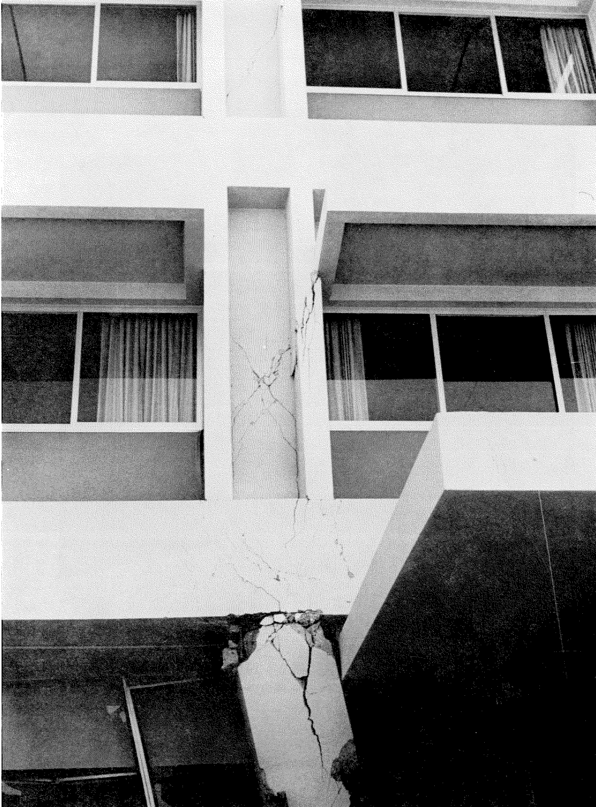
Figure 3.30 Above main entrance of Olive View Hospital. View showing cracks in second and third story of west wall of south wing.
