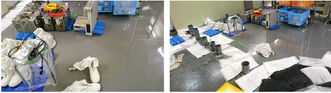
Fig. 3. Spring water leaking on the floor in the PSL room. (Left) The entire floor of the room was wet. (Right) Pipes were placed at the leaking points on the floor to prevent the water from spreading further. Water-absorbing sheets are also seen. The legs of the optical table can be partially seen on the top right. The photographs were taken in March 2015.
