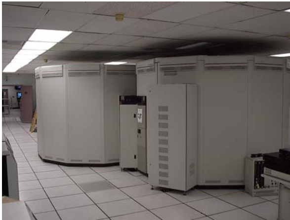
Figure 4. Tertiary storage tape silos at USC.
