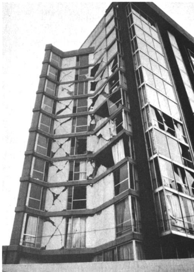
Fig. 4. Cracked masonry infills.
