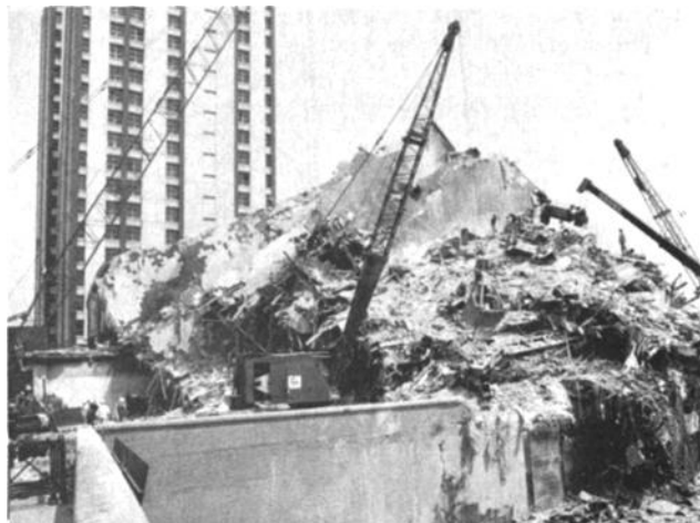
Fig. 5. Toppled tower at Pino Suarez.
