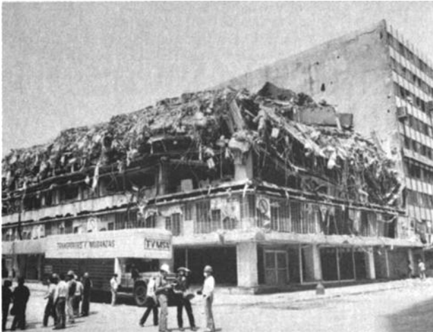
Fig. 6. Upper story collapse.
